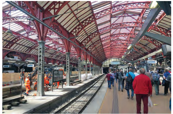
The impressive wooden vaulted ceiling in Copenhagen’s Central Railway Station, dating from 1911. Just like the UK, weekends often mean line closures and a team is replacing the track to the left
